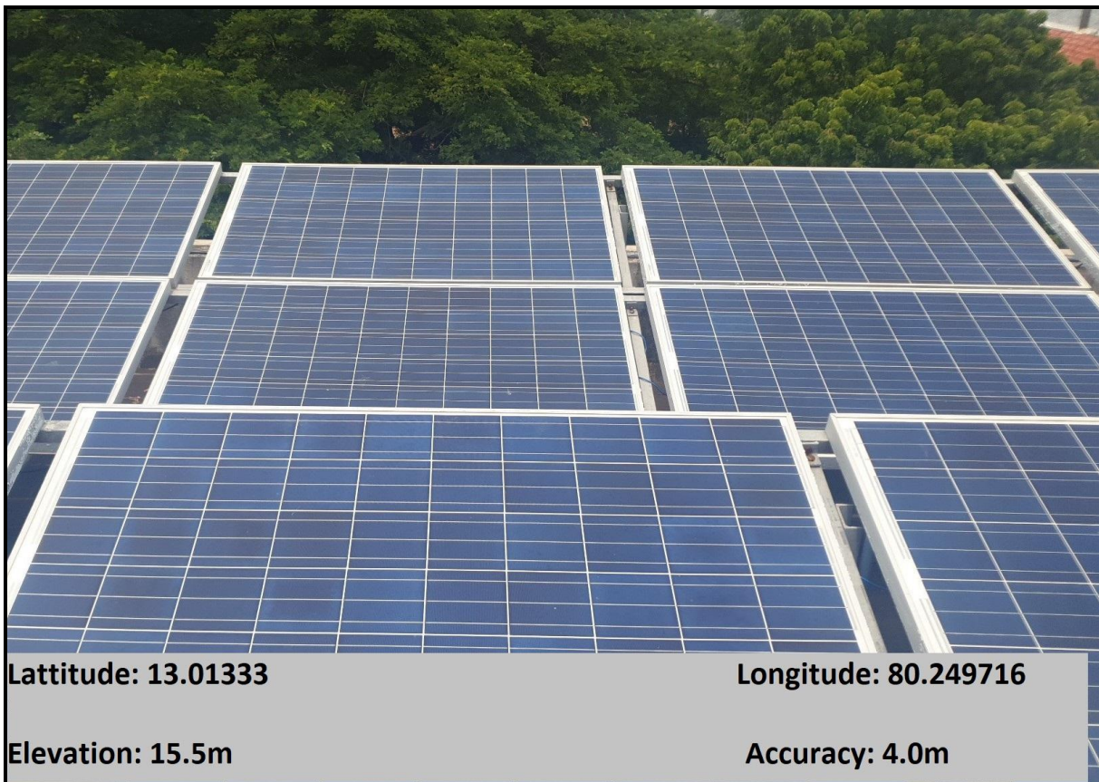
Solar Panels – B Block
